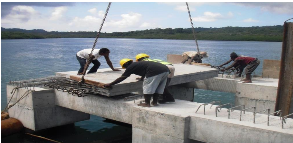
Figure 13: Fixing precast concrete decking on pile cap (PPE violations noted)
