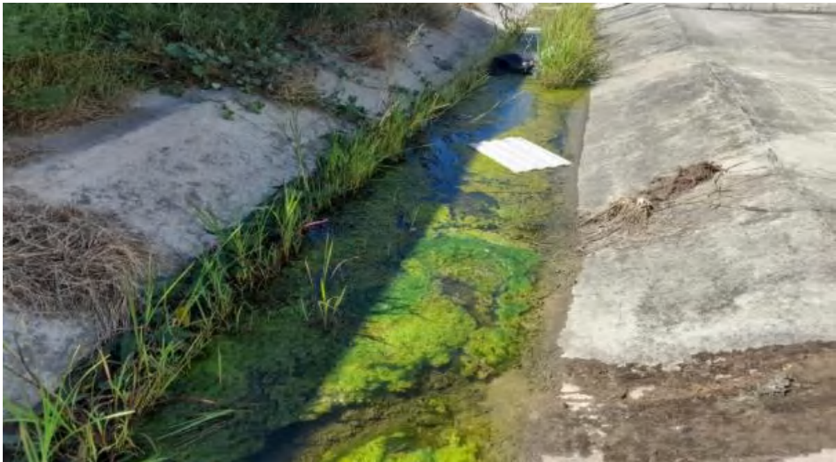
Figure 3.4. Storm water channel on the western side of the site. Storm water from the higher ground behind the building flows through this channel to the main drainage
