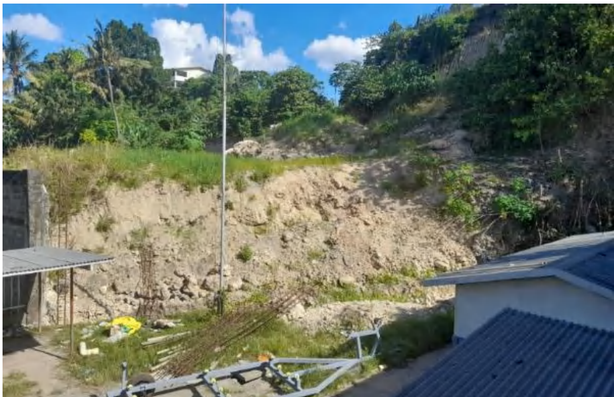
Figure 3.2. Collapse fencing and wall at the eastern side of the NMS compound
