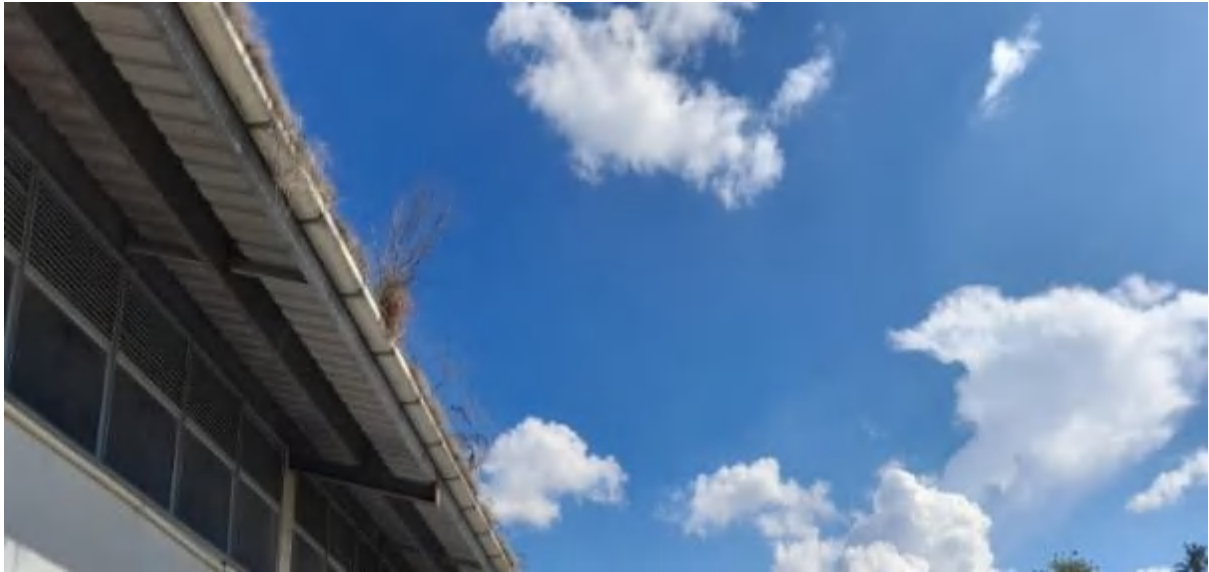
Figure 3.7. Grass and weeds growing in the rain gutters
