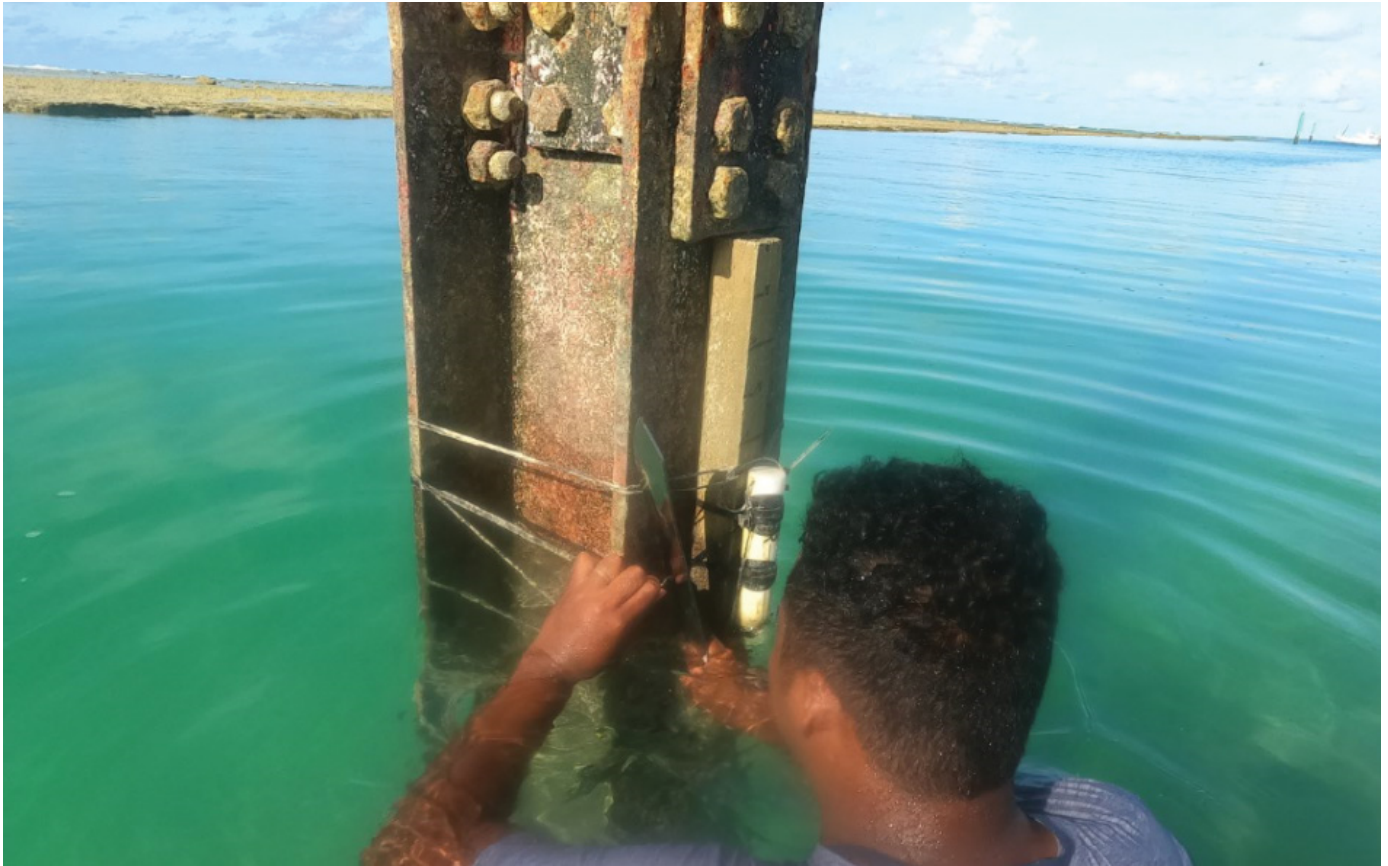
Figure 10: Example of a pressure sensor installation to monitor water levels in Nui, Tuvalu
