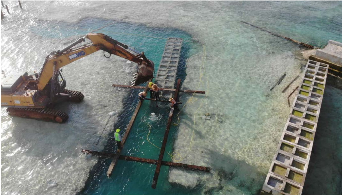
Figure 15: Use of working corridors and containment areas in Nukulaelae, Tuvalu
