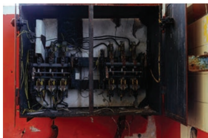
Asbestos ropes and backing board in circuit board
