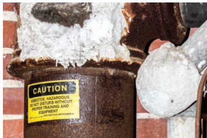
Pipe insulation (sprayed-on type)
