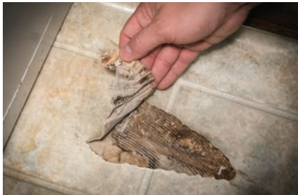
Adhesives below vinyl flooring
