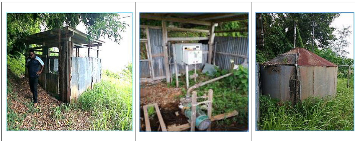
Plate 4-13: Pumping station and 0.015 ML suction tank in Tulagi
