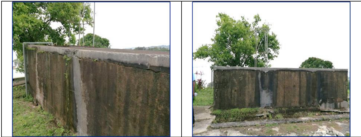
Plate 4-14: 0.05 ML high-level storage tank in Tulagi
